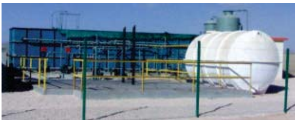
Fluidised media reactor
