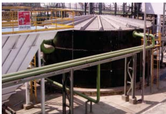
Fluidised media reactor
