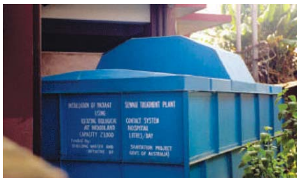
New generation packaged sewage treatment plant
