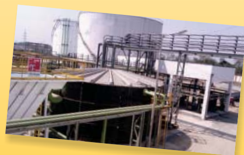
Moving bed bio-reactor
