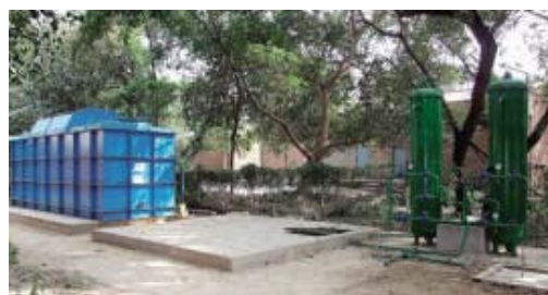
New generation packaged sewage treatment plant
